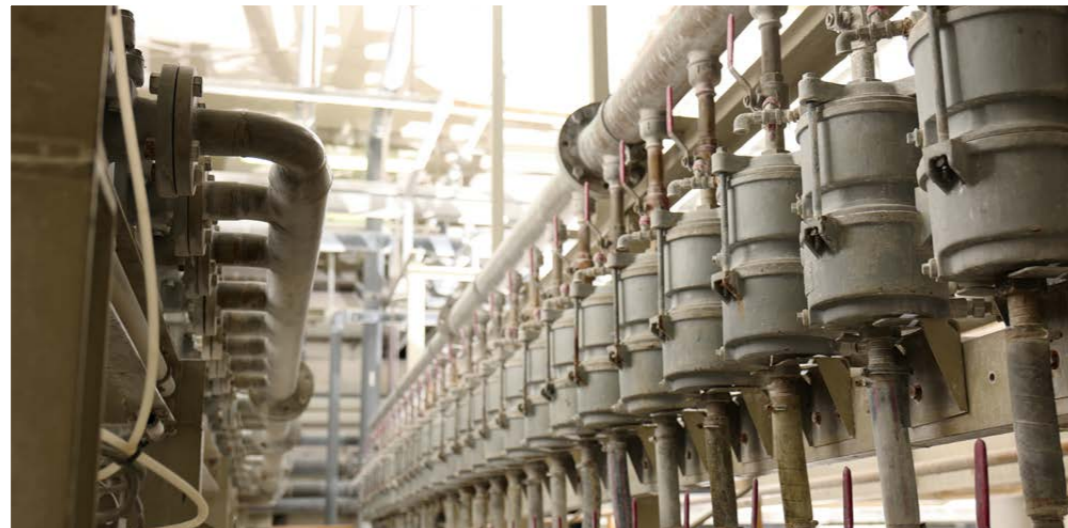
Separation of the sand particles and classification into different grain sizes by hydrocyclones
